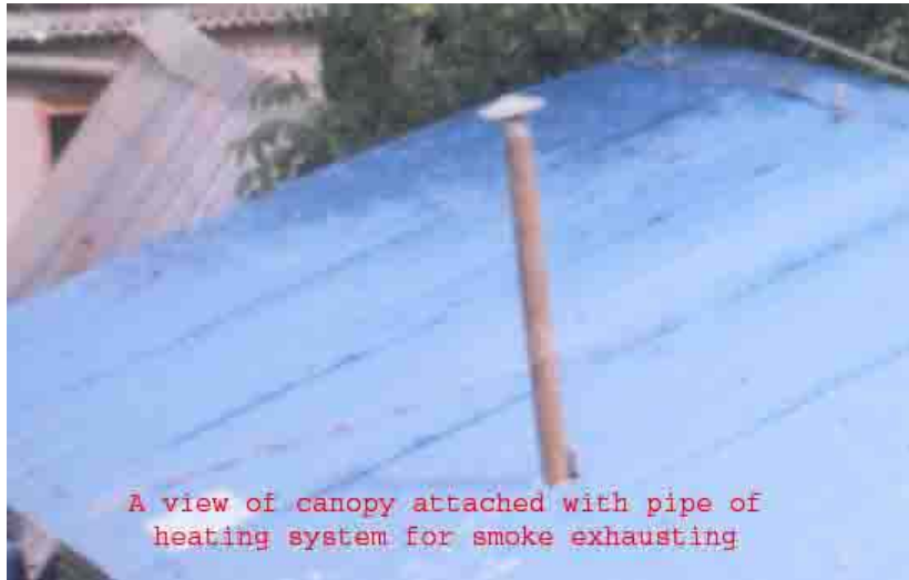
Heating systems is exhausting the smoke from one of shelter
